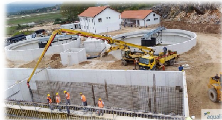
Waste water treatment plant (Montenegro)
